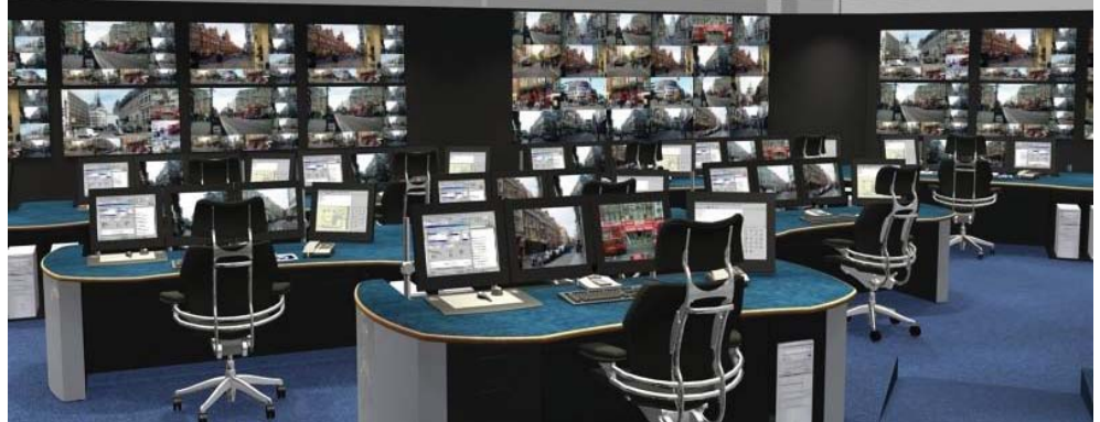
Central control room
